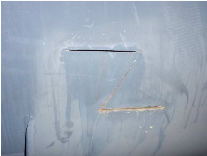
Figure 9: Damaged area on tank for leak simulation
